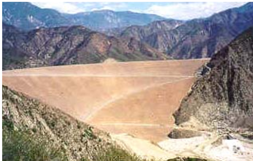
Photo from County of San Bernardino Department of Public Works- Flood Control District website at www.co.san-bernardino.ca.us/flood/damage
